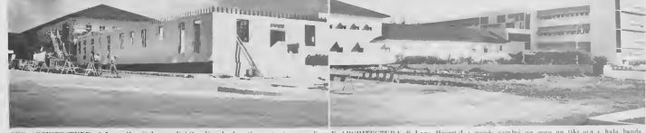
THE ARCHITECTURE of Lago Hospital was slightly altered when the east wing was dismantled recently. The operating section B, housed patients until 1953. After that, it was used for specialist offices. Section B's facilities have been relocated in the newly-air-conditioned section of the hospital. At right is a new view formerly blocked by the section.
